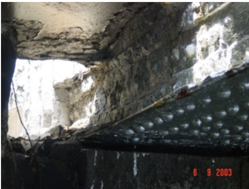
Fig. 3: Corrosion at bottom chord of lattice girder at the support (newly painted)
