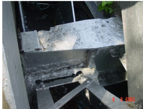
Fig. 4: Corrosion at connection of cross girder and main lattice (newly painted)
